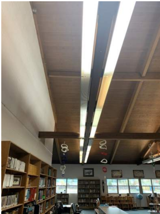
E10: Lighting lens discoloration in the Library
