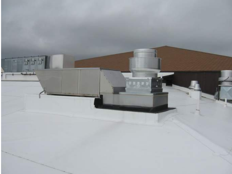
M11: Kitchen Makeup Air and Exhaust Fan
