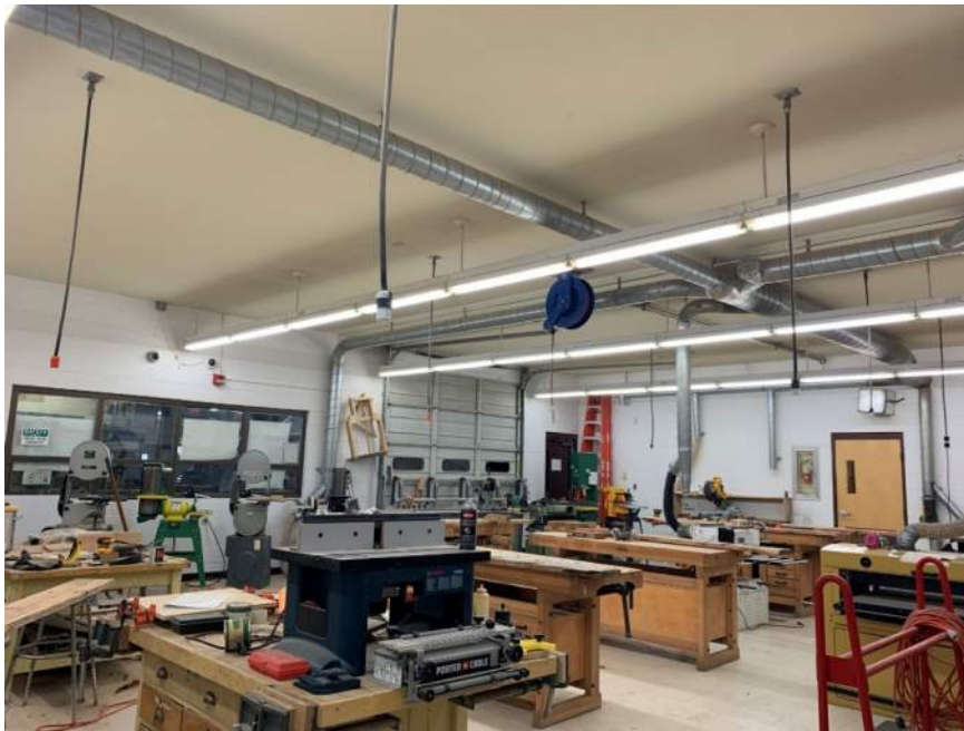
E8: Image of lighting in wood shop. Wire Guards are recommended.
