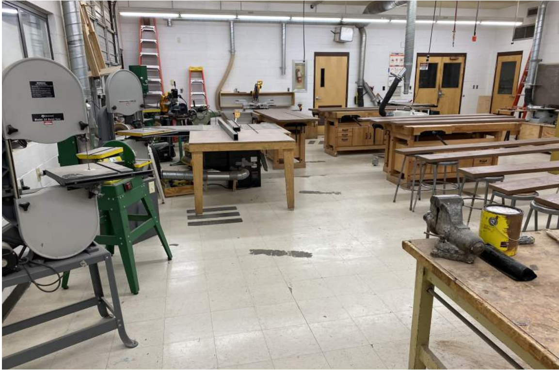
Another view of the shop space. Flooring and tables are worn as expected. The users of this space report slick floor surfaces when covered in sawdust.
