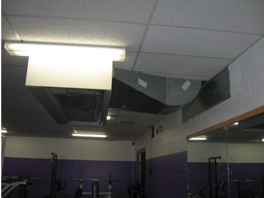
M9: Weight Room Fan Coil
