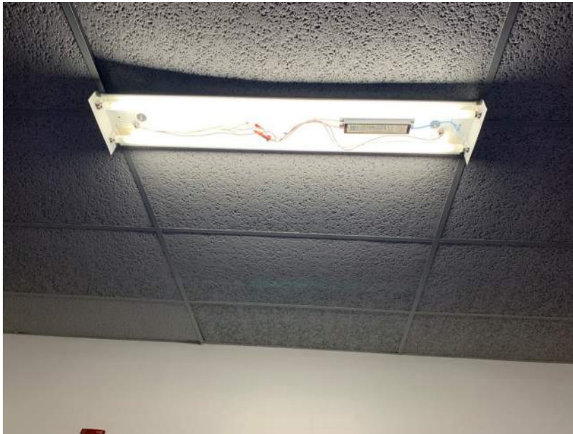
E12: Light in Locker room missing lens
