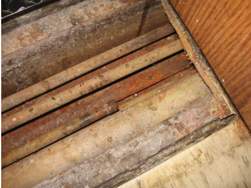
M17: Science Room Trench Piping
