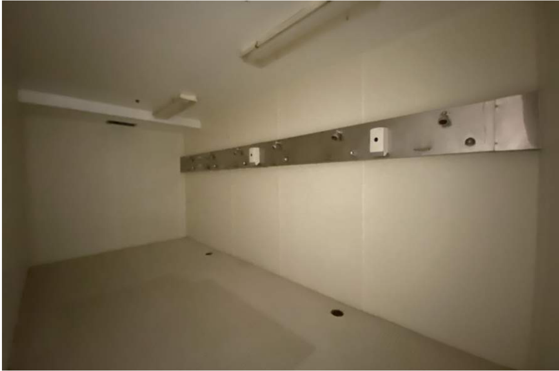
Gang showers in the lower level locker rooms are no longer designed in schools due to bullying and body shaming issues.
