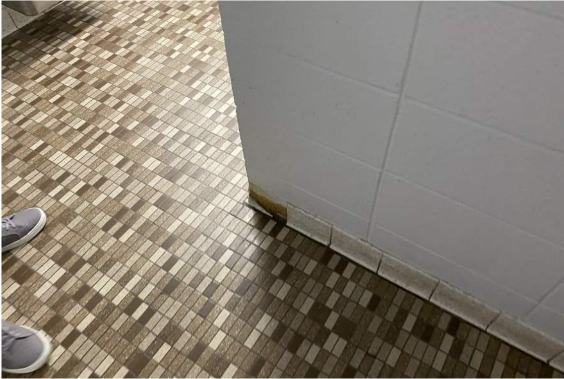
Most restrooms were in good condition, with minor areas of repair needed. However, this CMU block wall makes accessibility difficult for wheelchair users.
