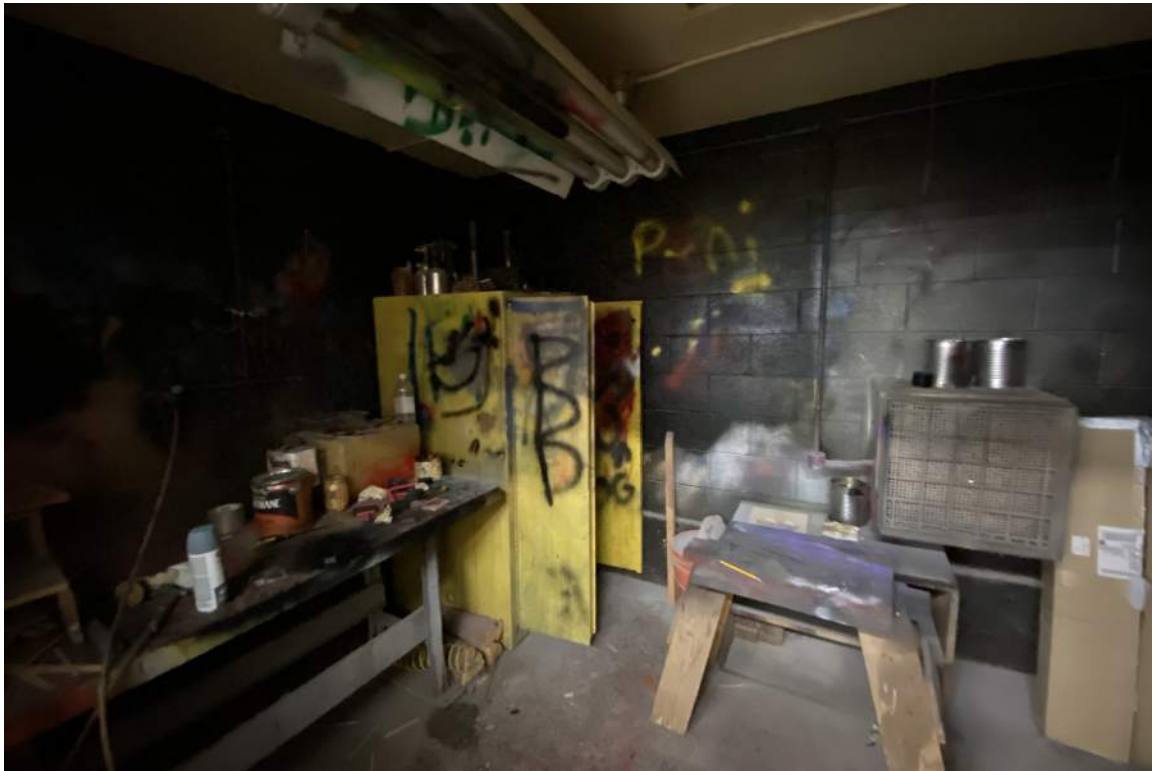
Spray booth in the CTE space. Problems of overspray are reported.
