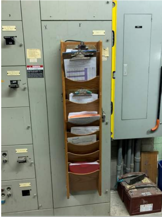
E3: File cabinet mounted to front of Motor Control Center
