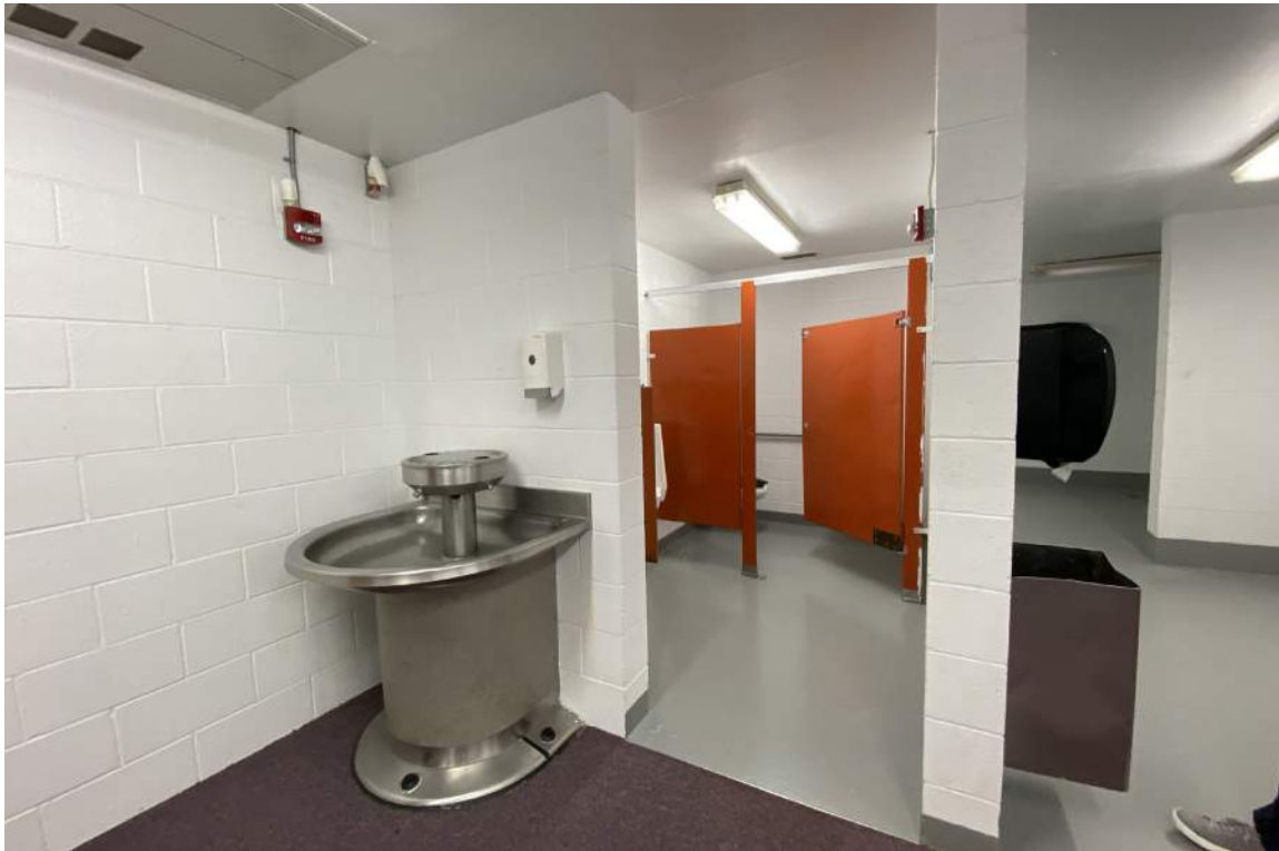
The main floor locker rooms with hand wash station. These stations are designed to serve students around its perimeter, but placement next to the CMU block wall limits access. This reduces the number of required lavatories per the International Building Code (IBC) and amendments per the Administrative Rules of Montana.
