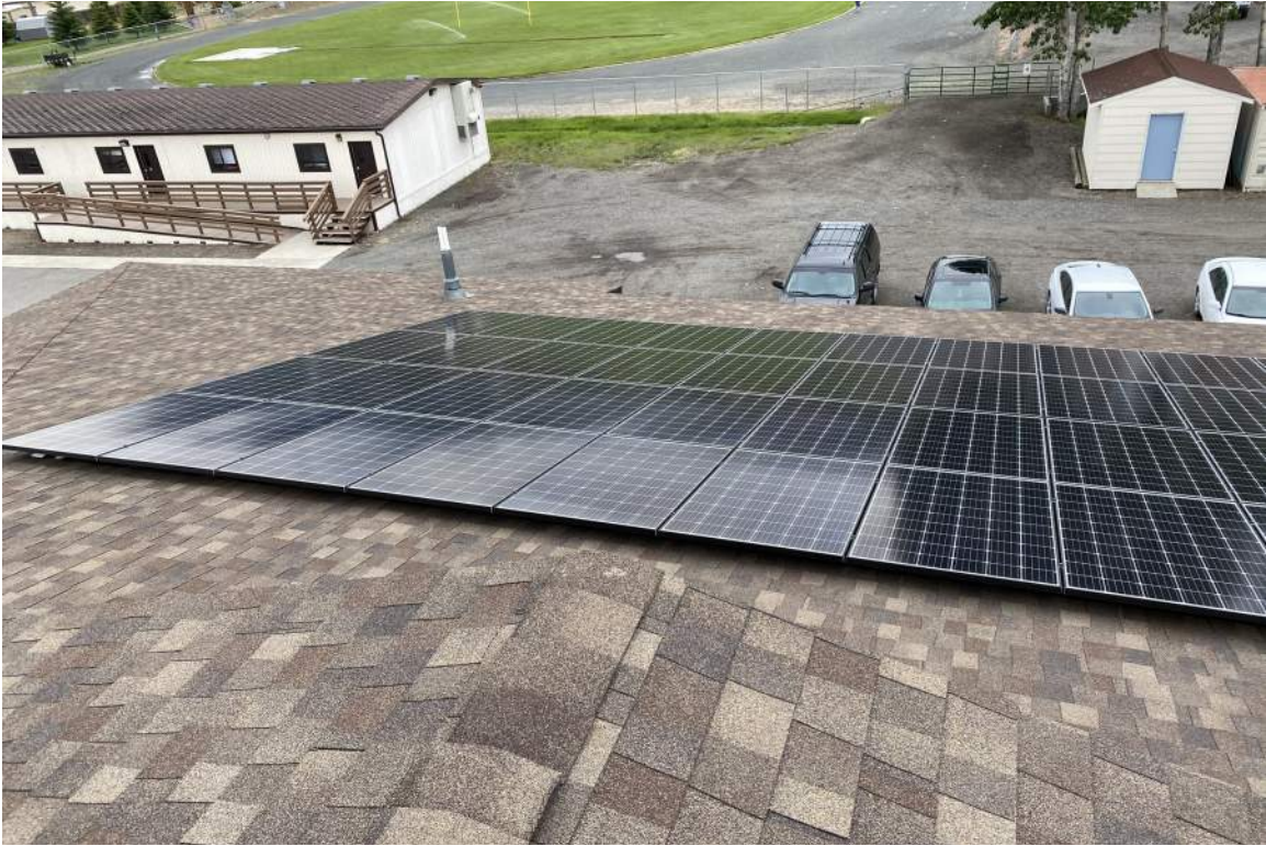
South Library roof, looking towards modulators and storage sheds. Shingles on the Library roof appeared in good condition. Modular roofs had shingles damaged and torn off, mostly from high winds over the previous weekend. Solar panels did not appear damaged.
