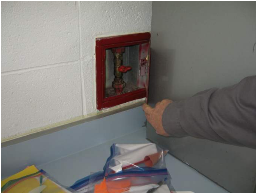
M18: Science Room Gas Shut Off
