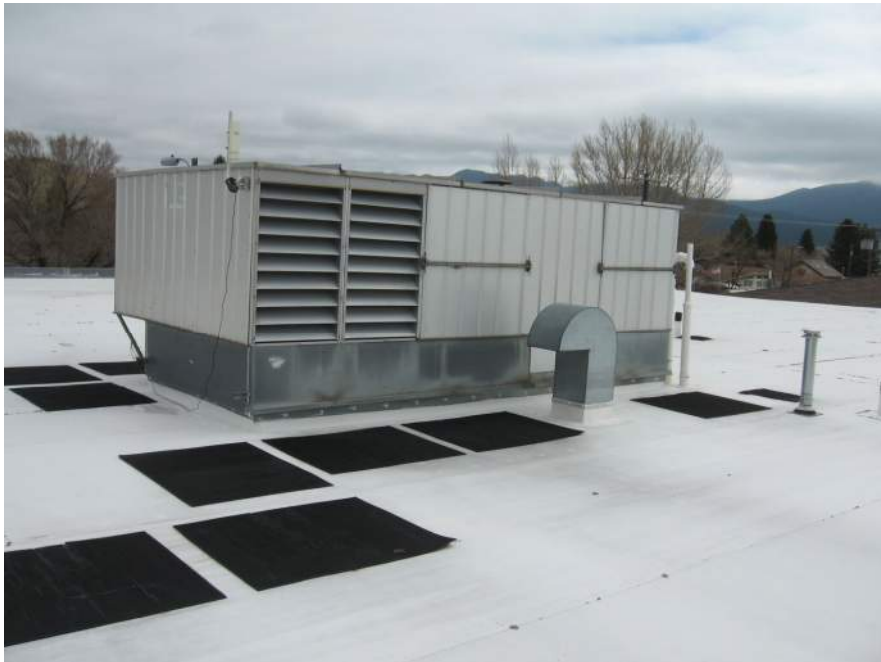
M12: Abandoned Rooftop Unit
