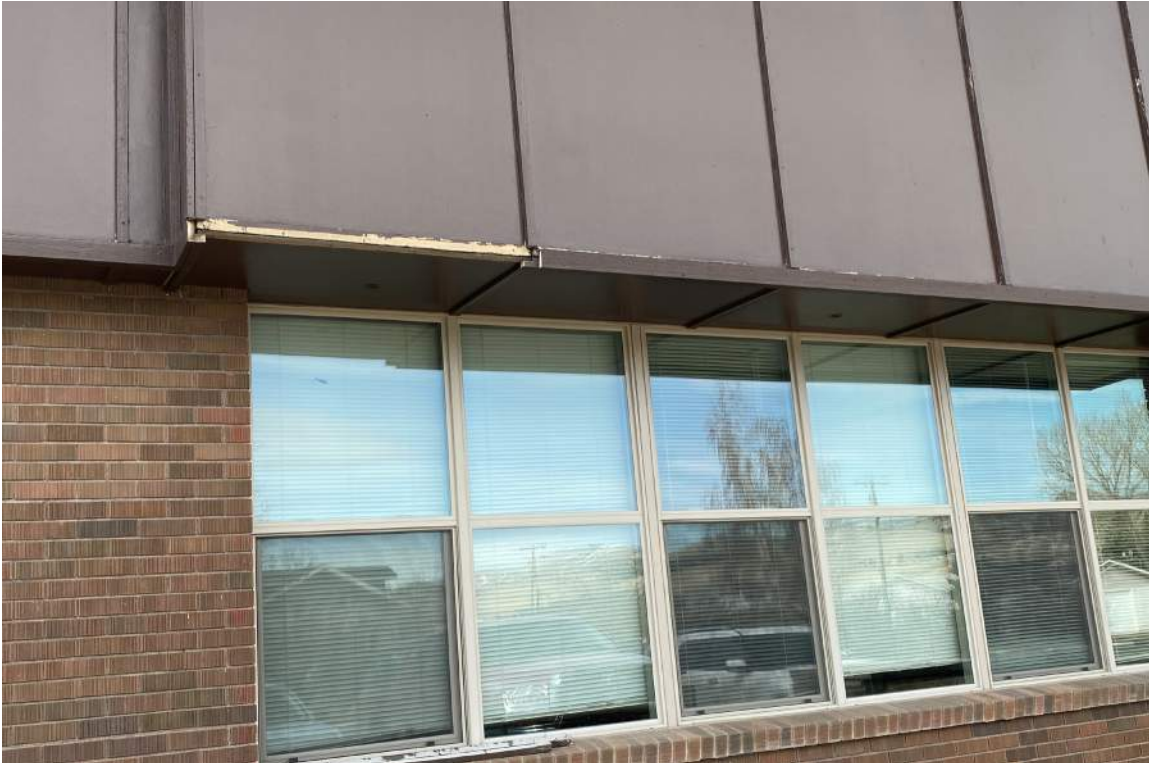
Wood fascia that is worn and coming apart.
