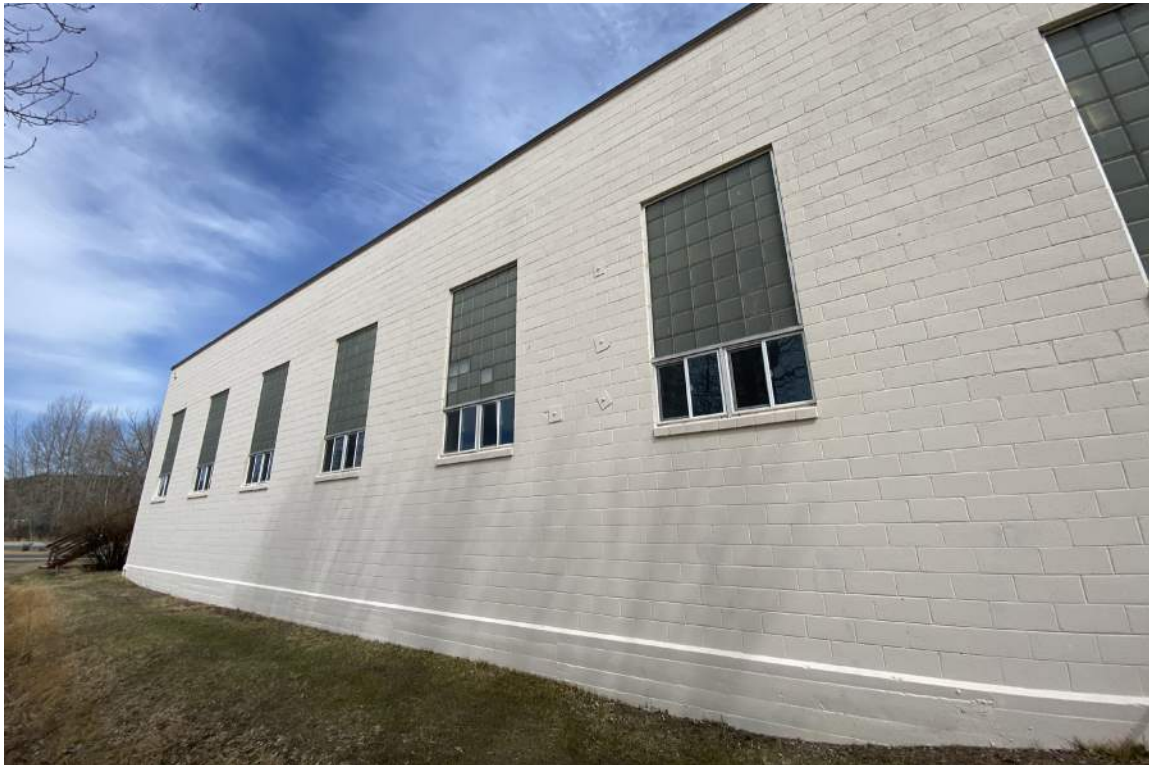
South side of Existing Gym, next to irrigation canal from the Boulder River. Masonry block is holding up well, and paint appears new.
