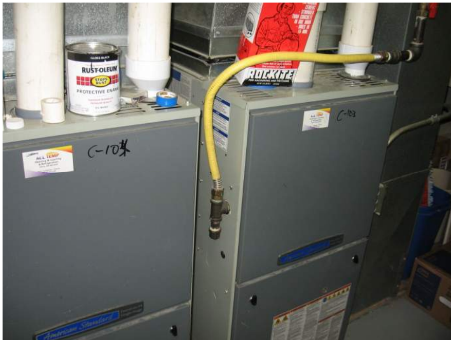
M14: Room C118 Furnace
