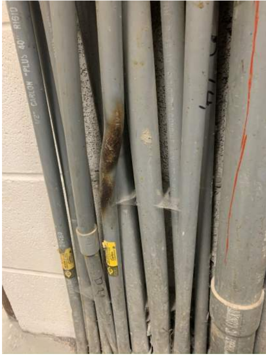
E5: Conduit shows signs of electrical fire and should be investigated by Electrician and replaced.
