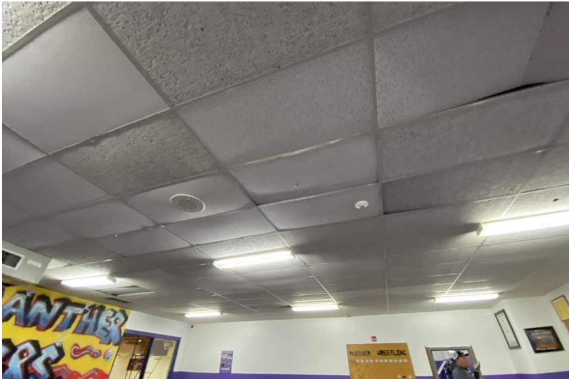
Ceiling tiles in the wrestling room are severely warped and discolored, from previous roof leaks and excessive moisture. Many areas in the school have the same issue and need to have the tiles replaced.
