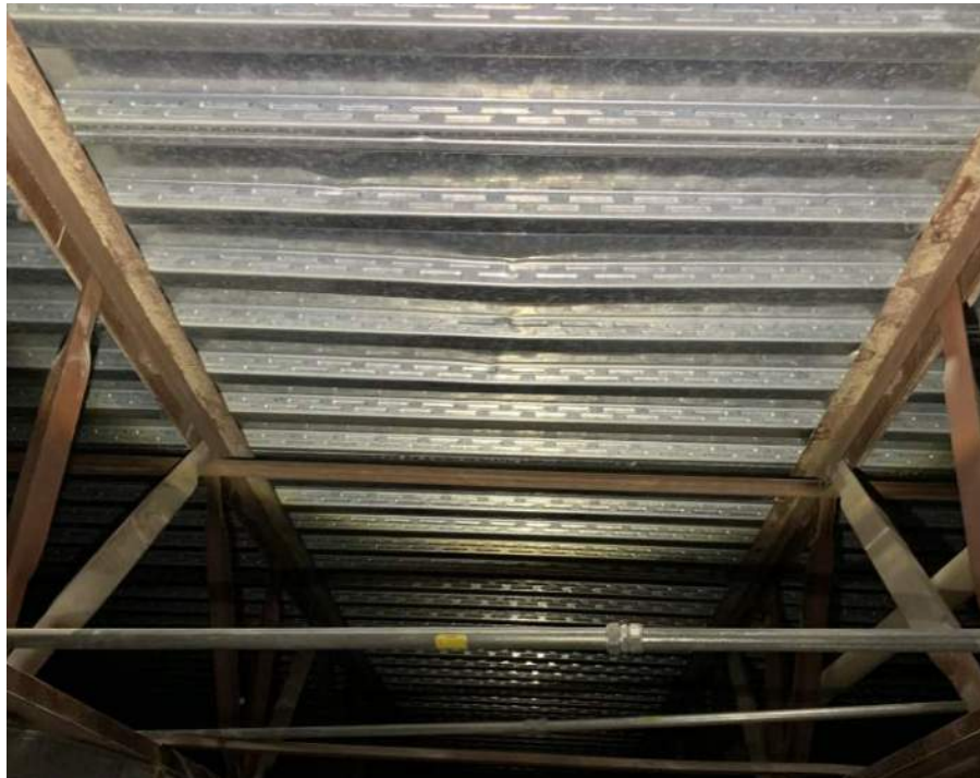
Figure 6. Deformed Metal Deck Below Weight Room (1985 Addition)
