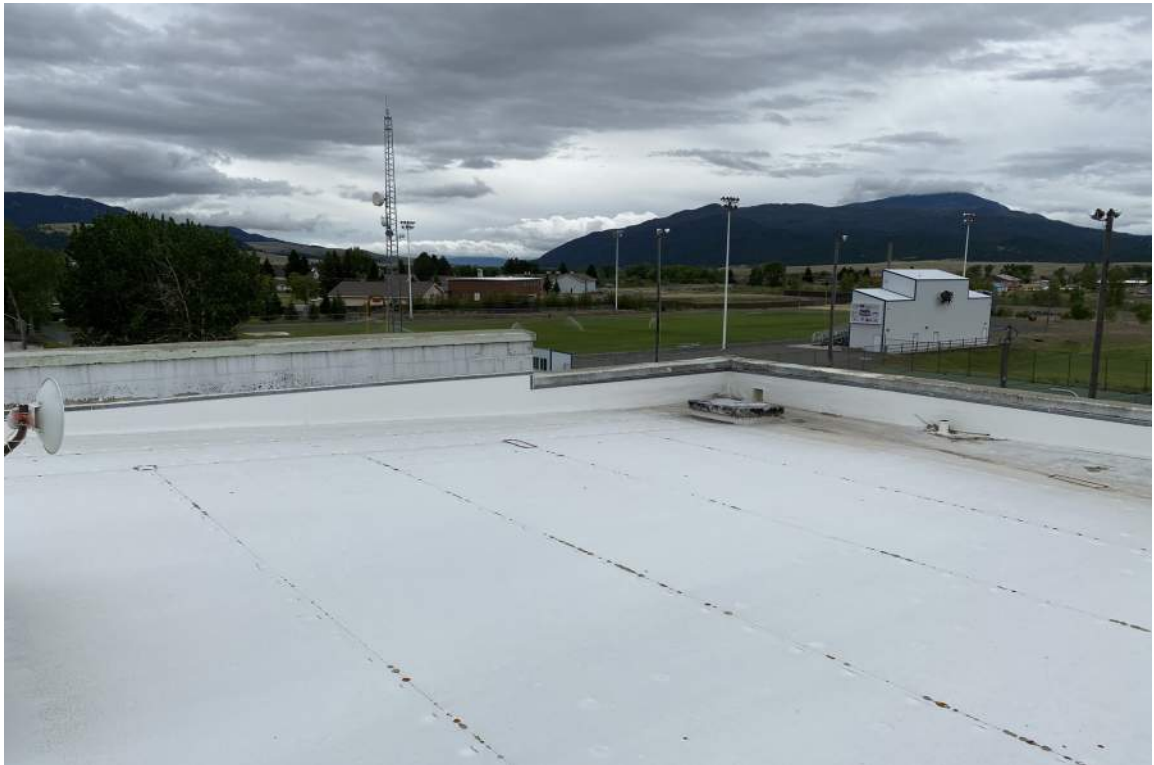
The majority of the existing roofs appeared to be in good condition. This roof, over the Existing (South) Gym, had very little damage and transitions and termination bars were in good working order.
