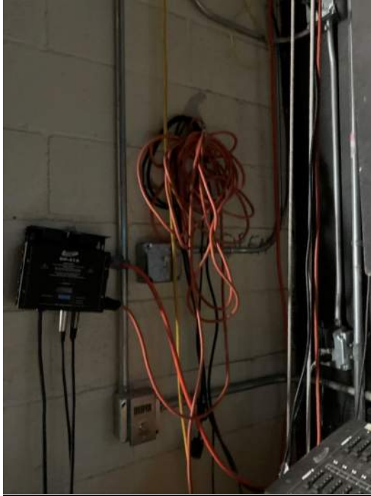
E7: Extension cords at stage area.
