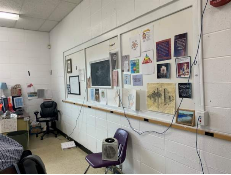
E13: Communication cable draped across teaching wall to desk.
