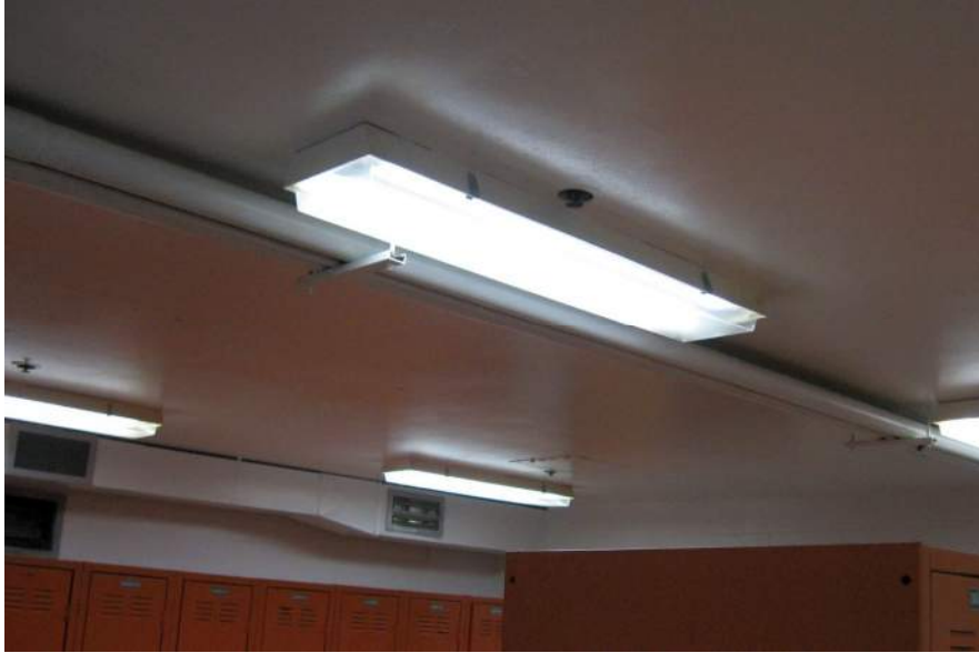
M7: Lower Level Locker Room Fire Sprinkler
