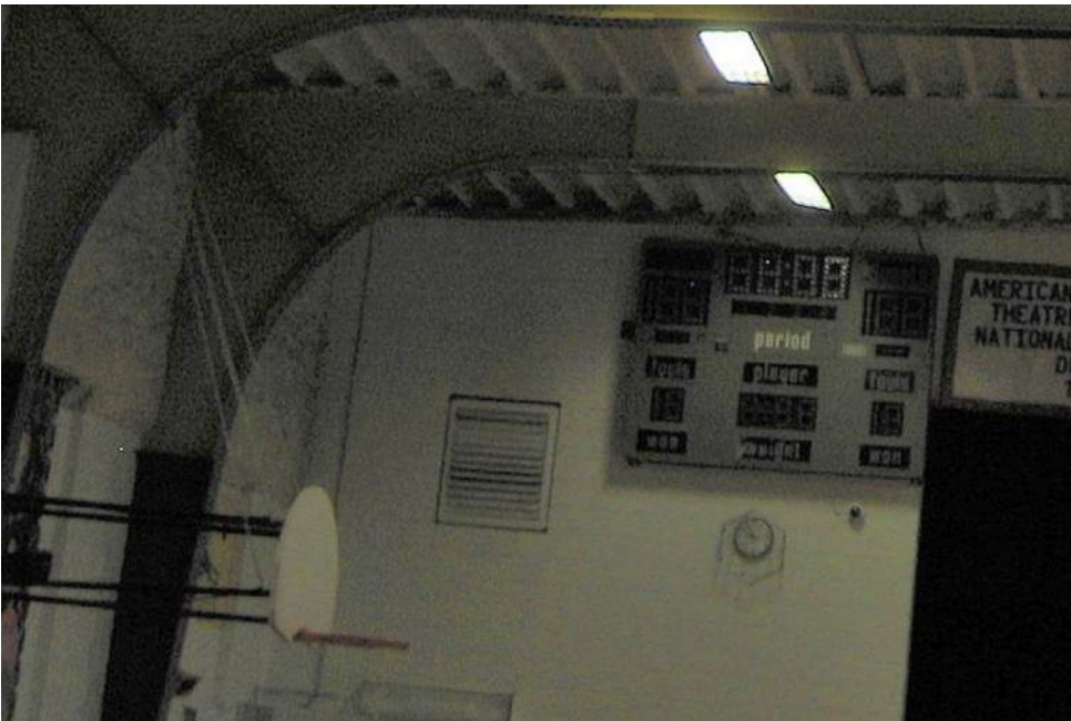
M2: Old Gym Unit Heater
