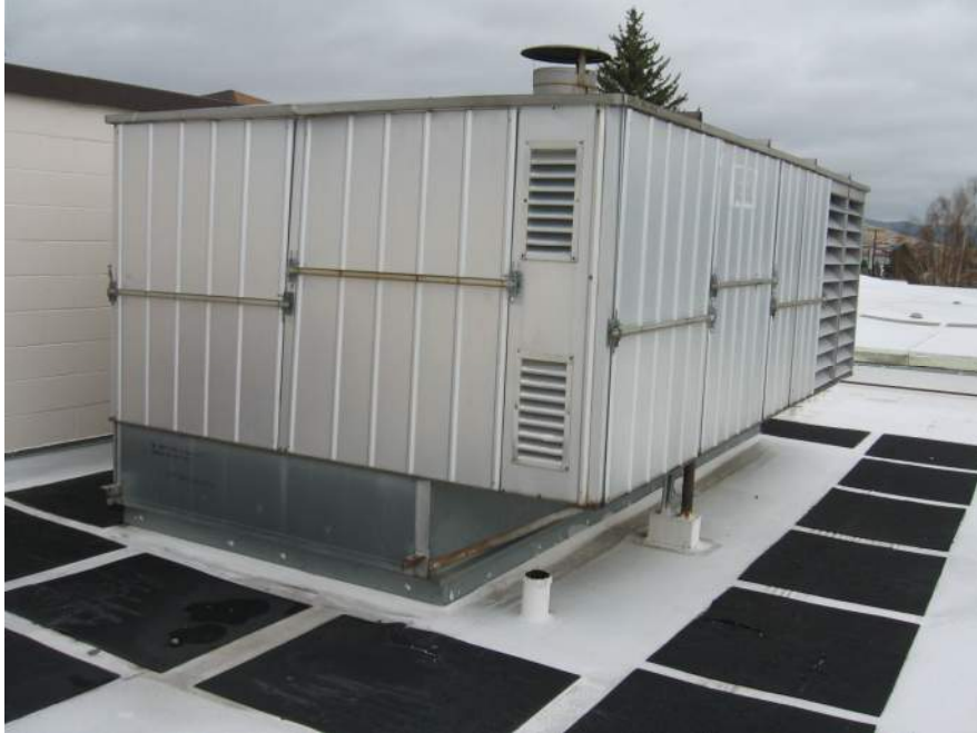
M19: Wood Shop Rooftop Unit
