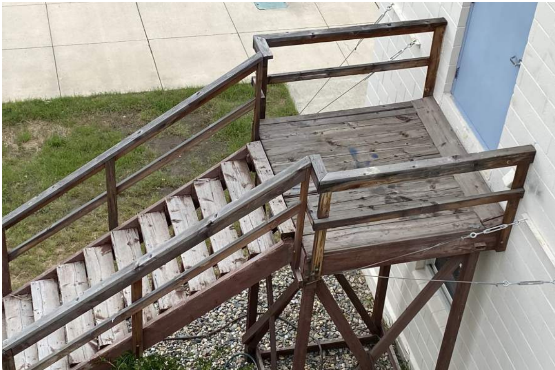
The egress stairs from the Art Room, as seen from the South Gym roof. The wood appears deteriorated and is secured to the building with cables. This stair does not comply with current accessibility codes and needs to be replaced with a more permanent stair.
