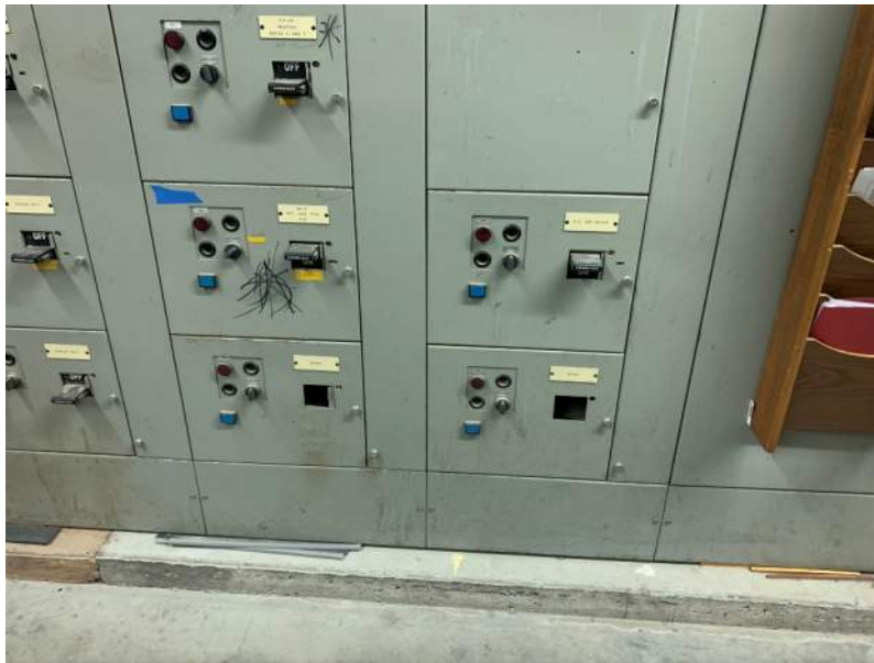
E2: Missing cover plates on MCC buckets need to be repaced.
