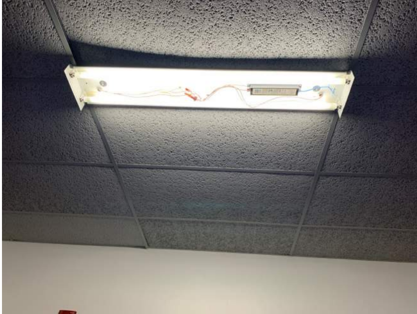
E15: Damaged fixture in weight room.
