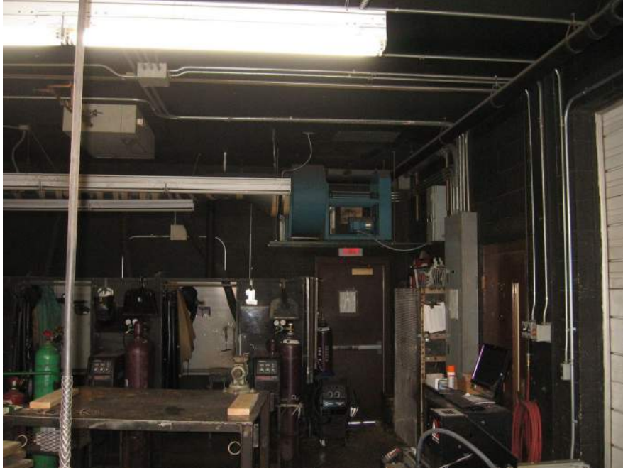
M21: Welding Shop Exhaust Fan
