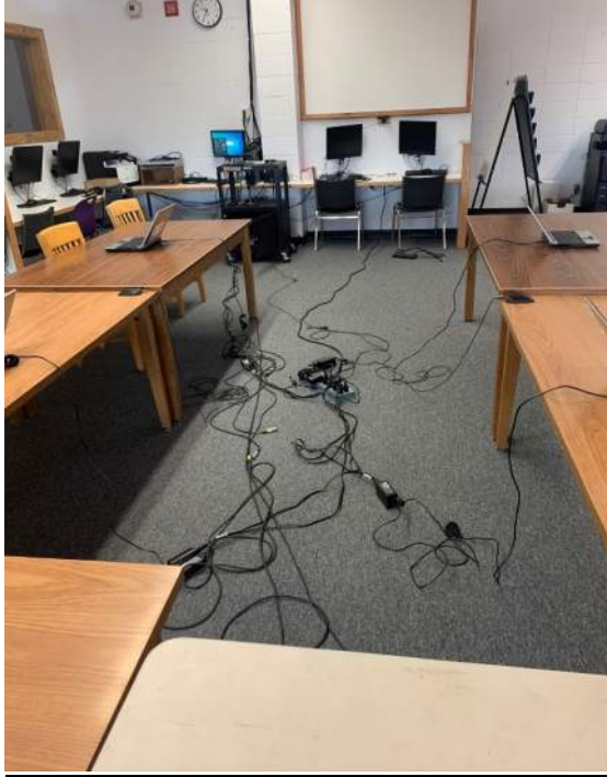
E11: Extension cords and power strips at meeting area in Library
