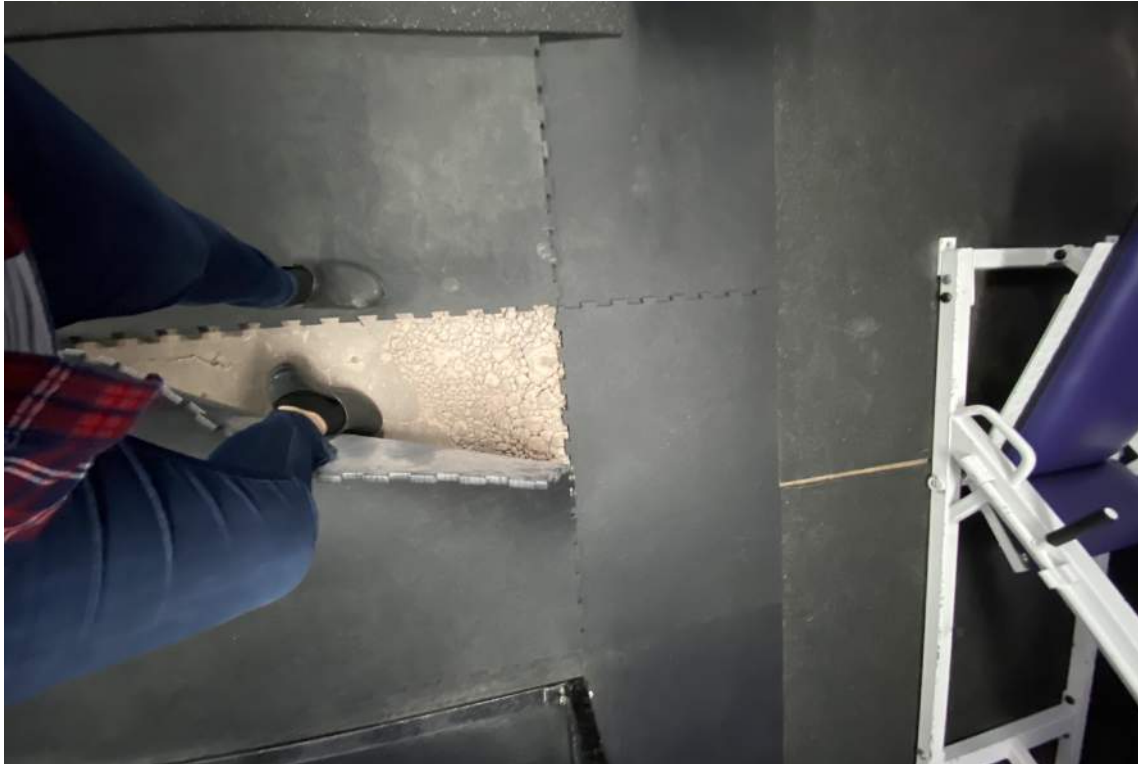
Crumbling composite concrete deck of weight room. Heavy plates and dropping of weights has resulted in severe deterioration of the deck. While this is not a structural problem, it is recommended that the weight room be moved to a floor with a thicker concrete slab.
