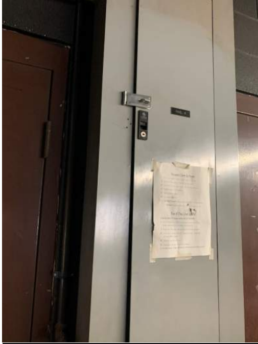
E9: Panel in Metal shop with door latch not properly working.
