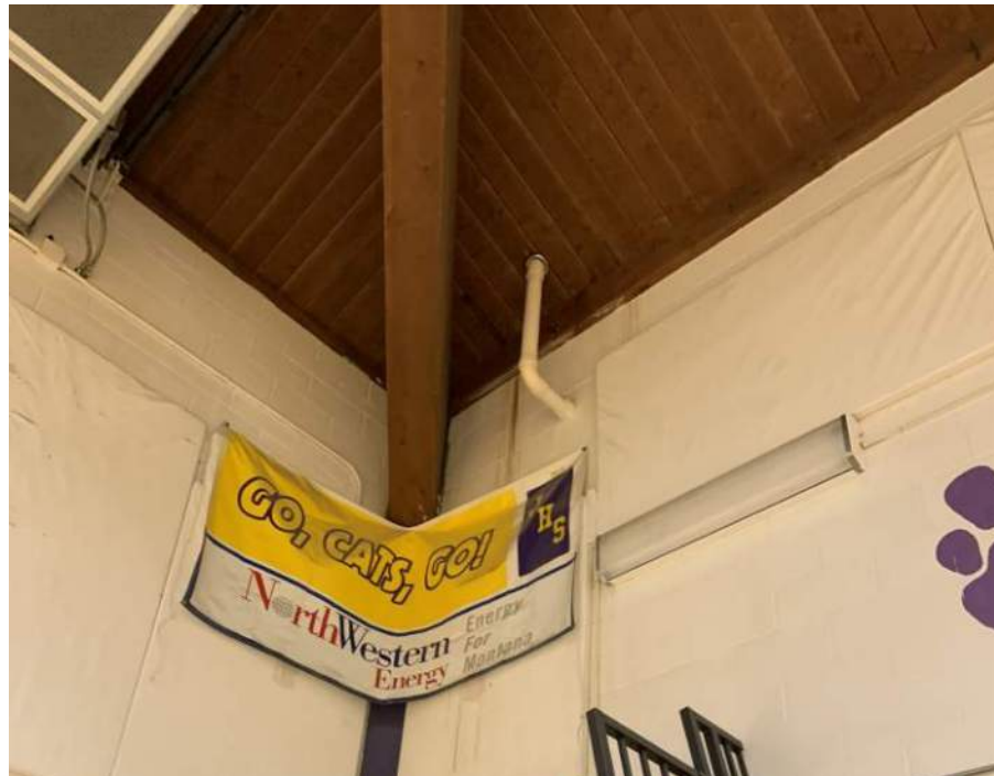
Figure 4. Water Stains on south CMU wall of 1985 Gym
