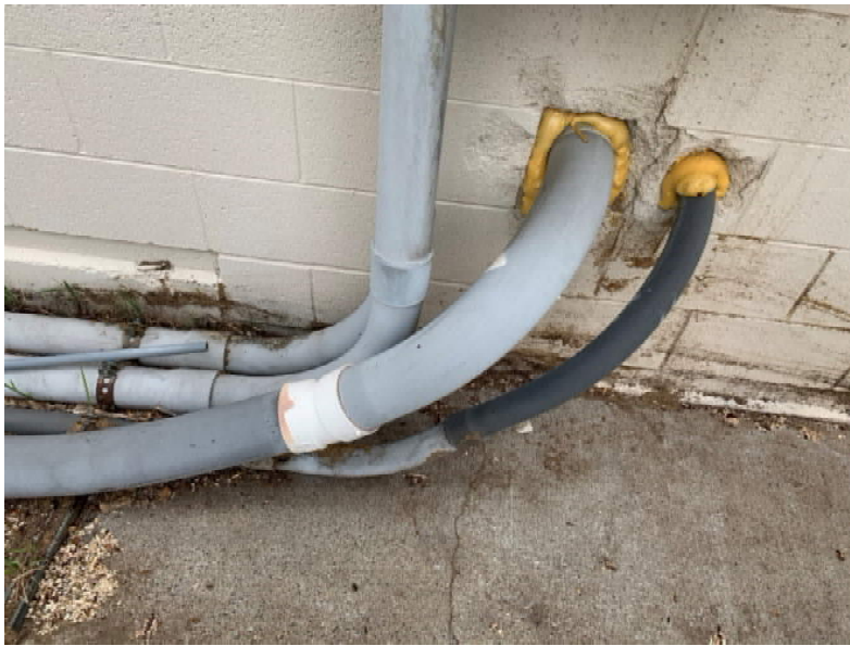
E4: Conduit entrance at dust collector. Shows change in materials at fittings, conduit runs and sealant used.
