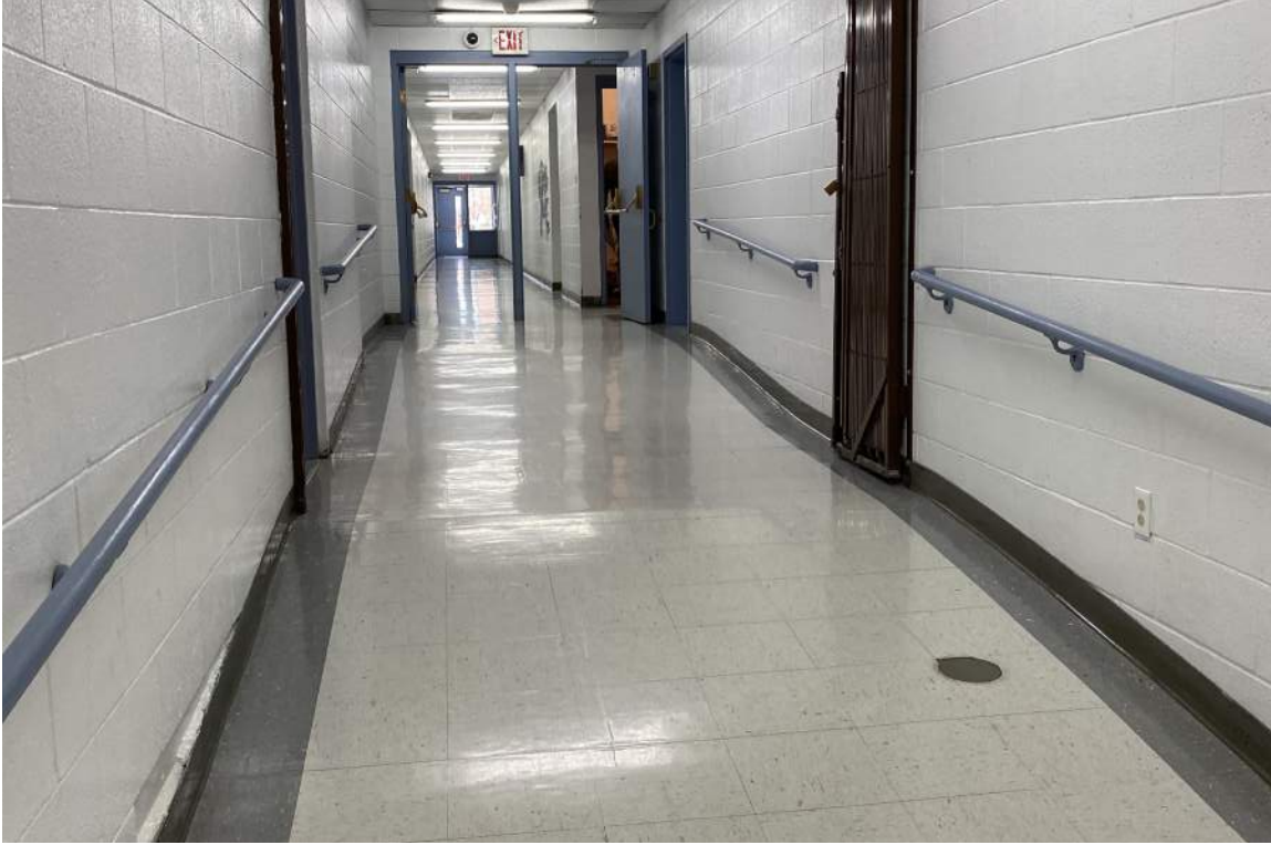
Ramps in main hallway running east-west. Landings, handrails, and slopes all appear to be within current ADA requirements.
