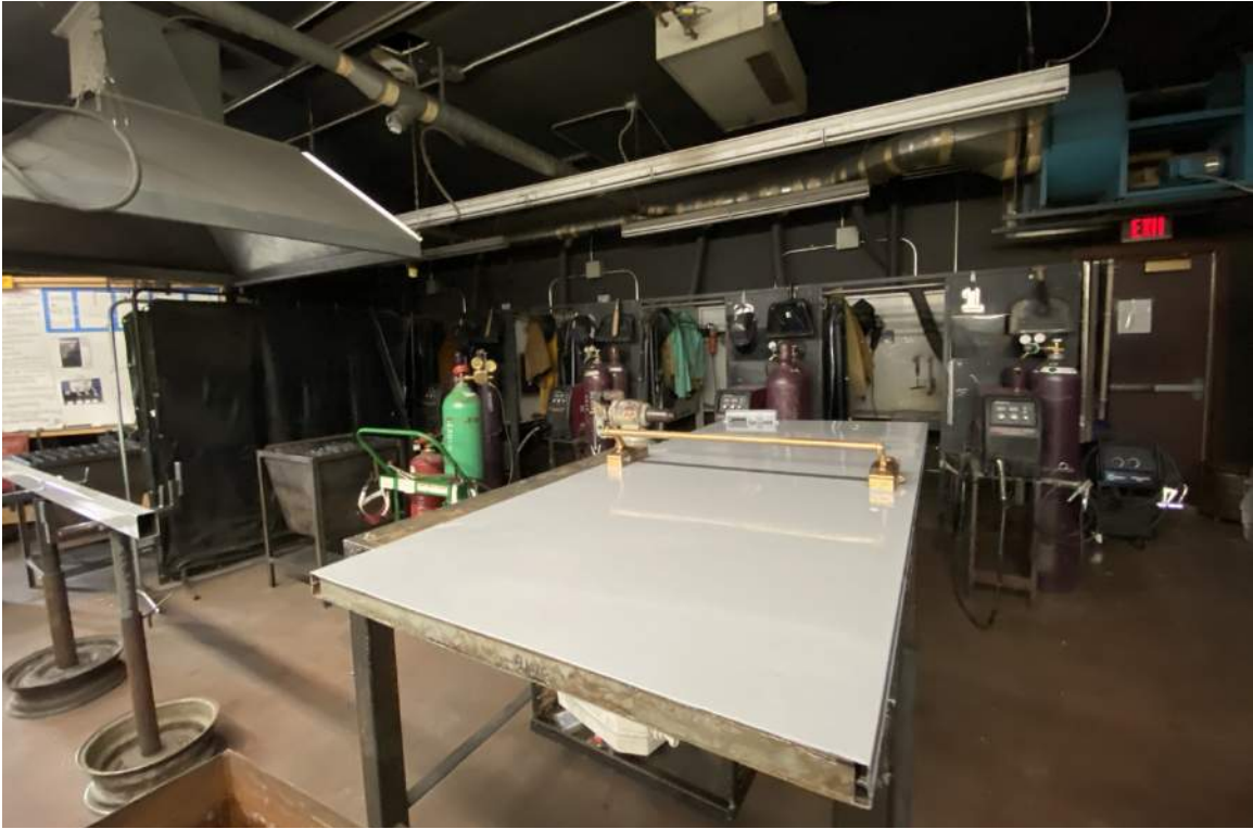
The welding space has a close proximity to the small engines space. Gas fumes are smelled in this room and there are questions of flammability.
