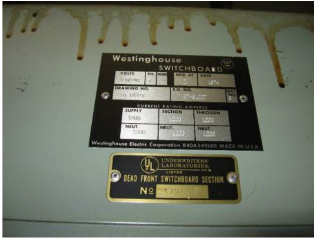
E1: Main Distribution Board showing liquid substance leaking from/onto equipment.
