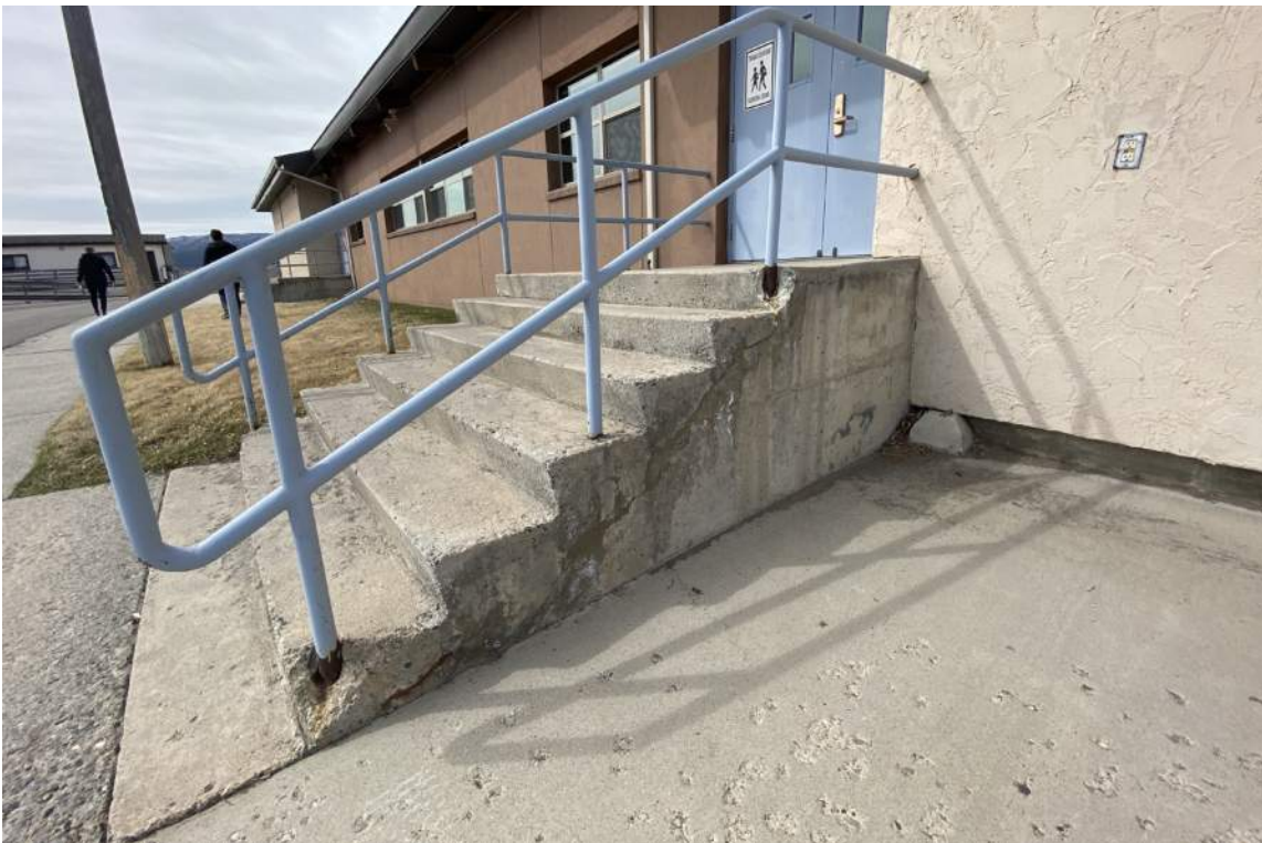
An area of spalling concrete around handrail posts. While not dangerous or against accessibility codes, continued wear will eventually lead to the handrail dislodging from the concrete. This could give way under lateral load when in use and cause injury.
