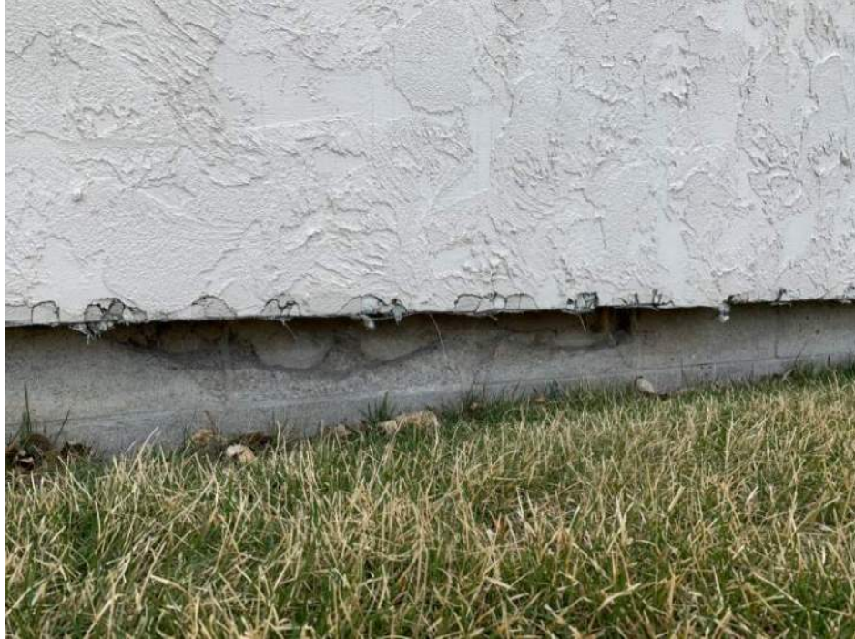
Figure 7. Exterior Foundation Wall Damage at 1985 Gym
