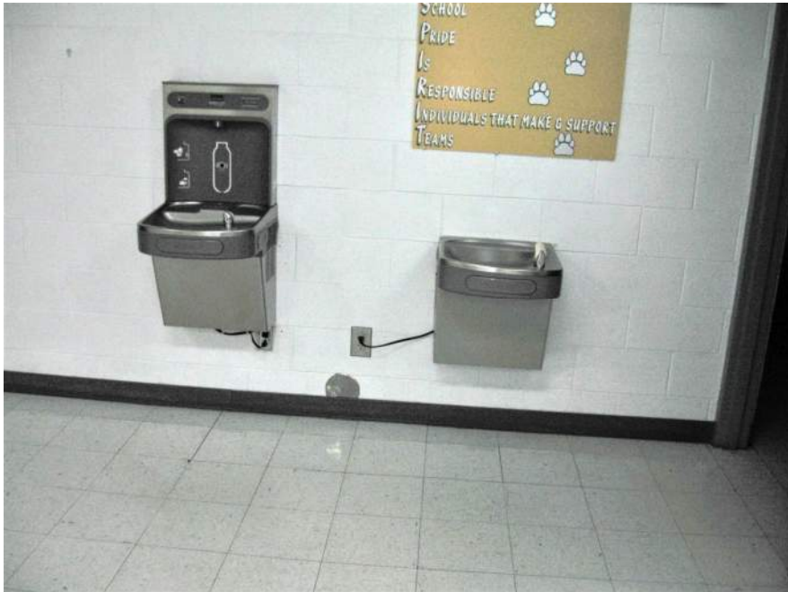
M10: Electric Water Coolers
