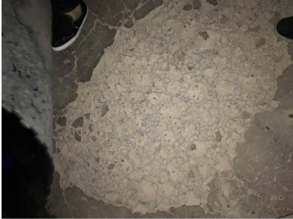
Figure 5. Deteriorated Concrete Floor Slab in Weight Room (1985 Addition)
