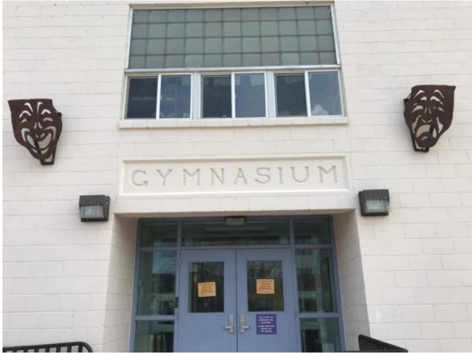
Figure 19. Cracking in Exterior Wall Around Plaque (1956 Addition)
