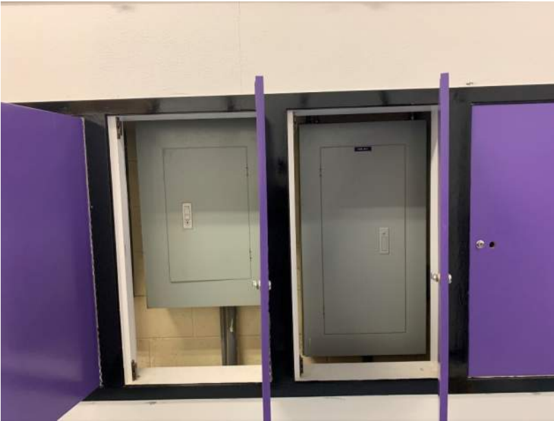
E14: Panels off of Gym lobby enclosed in cabinets. Working space clearances not met.
