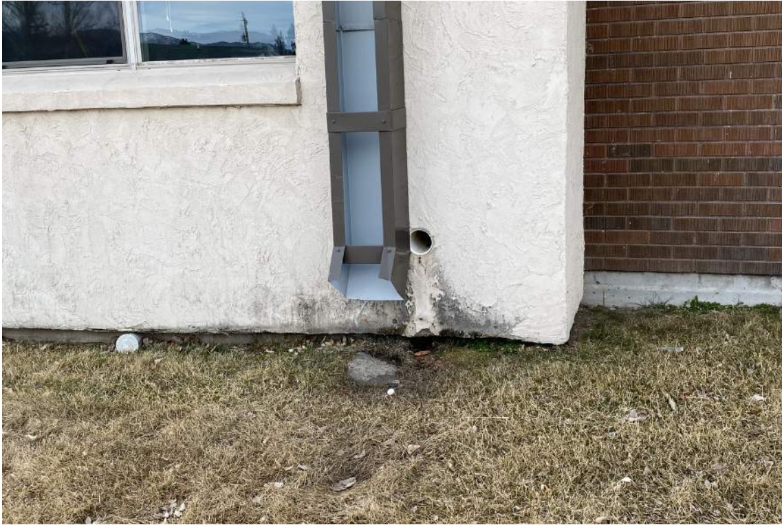
A large roof downspout and overflow on the north side of the building. Most of these large downspouts did not have a splash block or other method of diverting large quantities of water away from the foundation, and most runoff soaks into the grass area.
