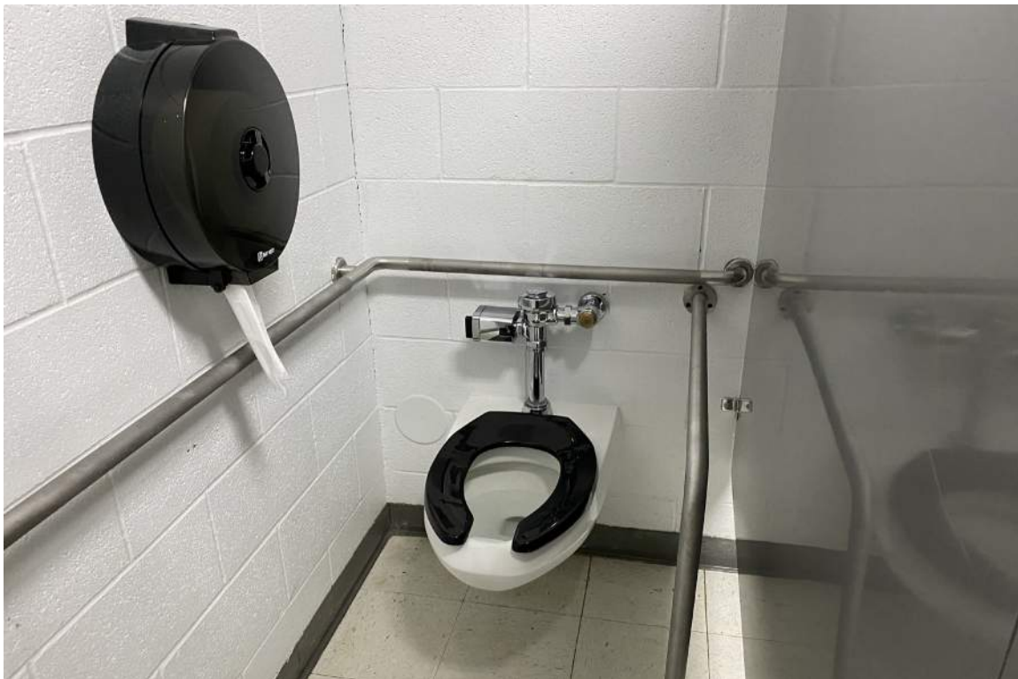
Toilet fixture and stall in restrooms adjacent to Cafeteria seating area. Even though it has several grab bars, this restroom, like most in the school, does not meet current codes for accessibility.
