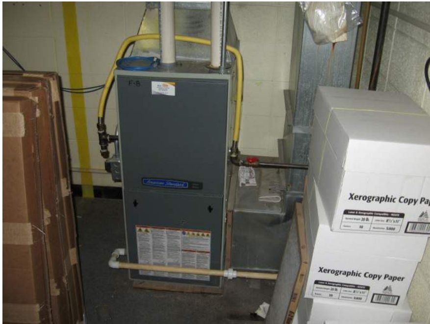
M13: Room C112 Furnace
