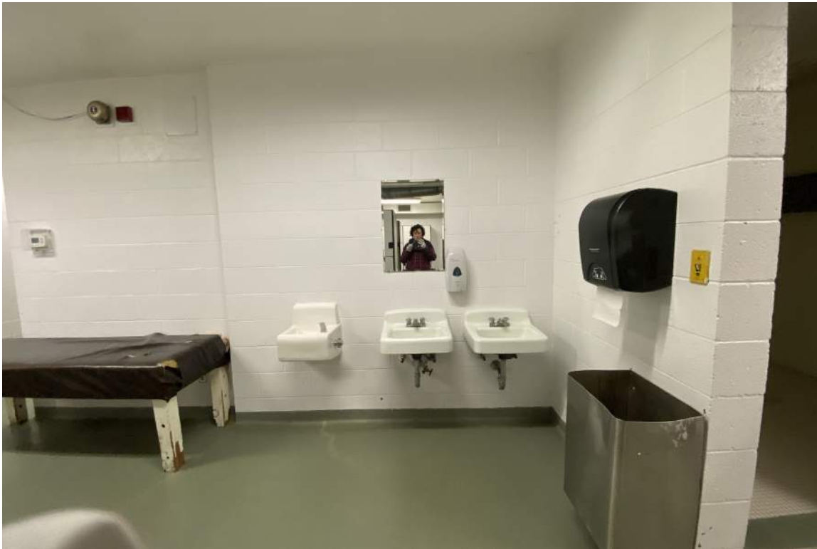
Women's lower level locker room. Floor and walls are in good condition but the training bench is very worn.
