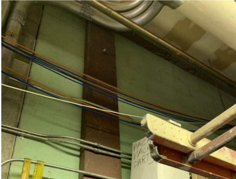
Figure 13. Channel Ledger and Column at Interface Between Mechanical Room and Wood Shop
