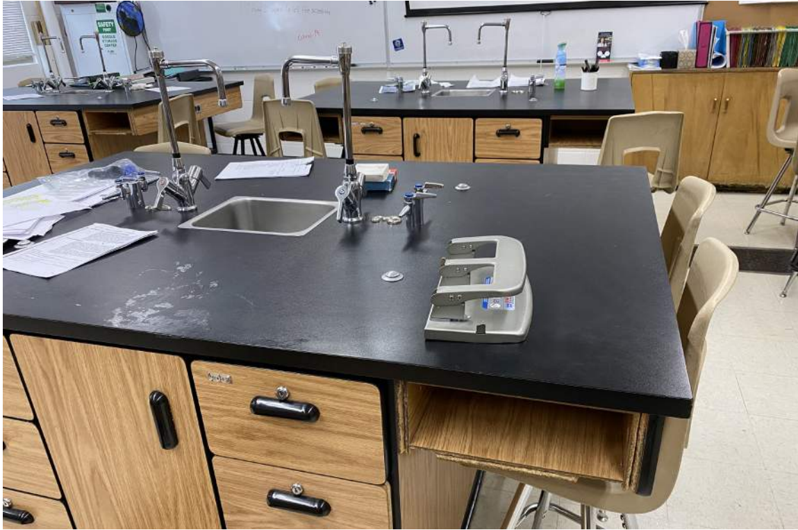
Casework and countertops in the Life Sciences room. While most of these are in good condition, there are areas of wear. This room is too small for a typical science room.
