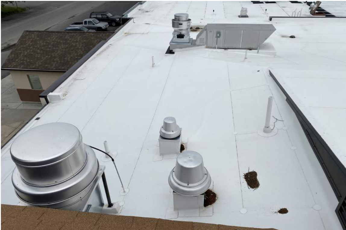
The roof looks relatively new. This area over the Kitchen space had welds and wrapping of membrane applied correctly.
