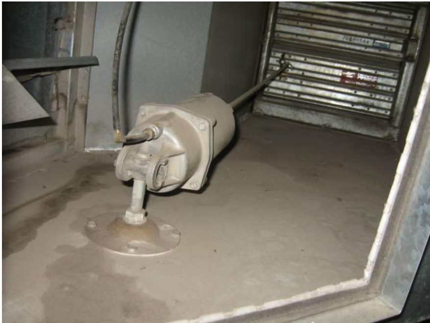
M16: Furnace Outdoor Air Pneumatic Damper
